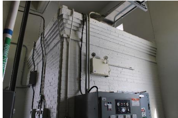
Plate 10: Brickwork at electrical room
